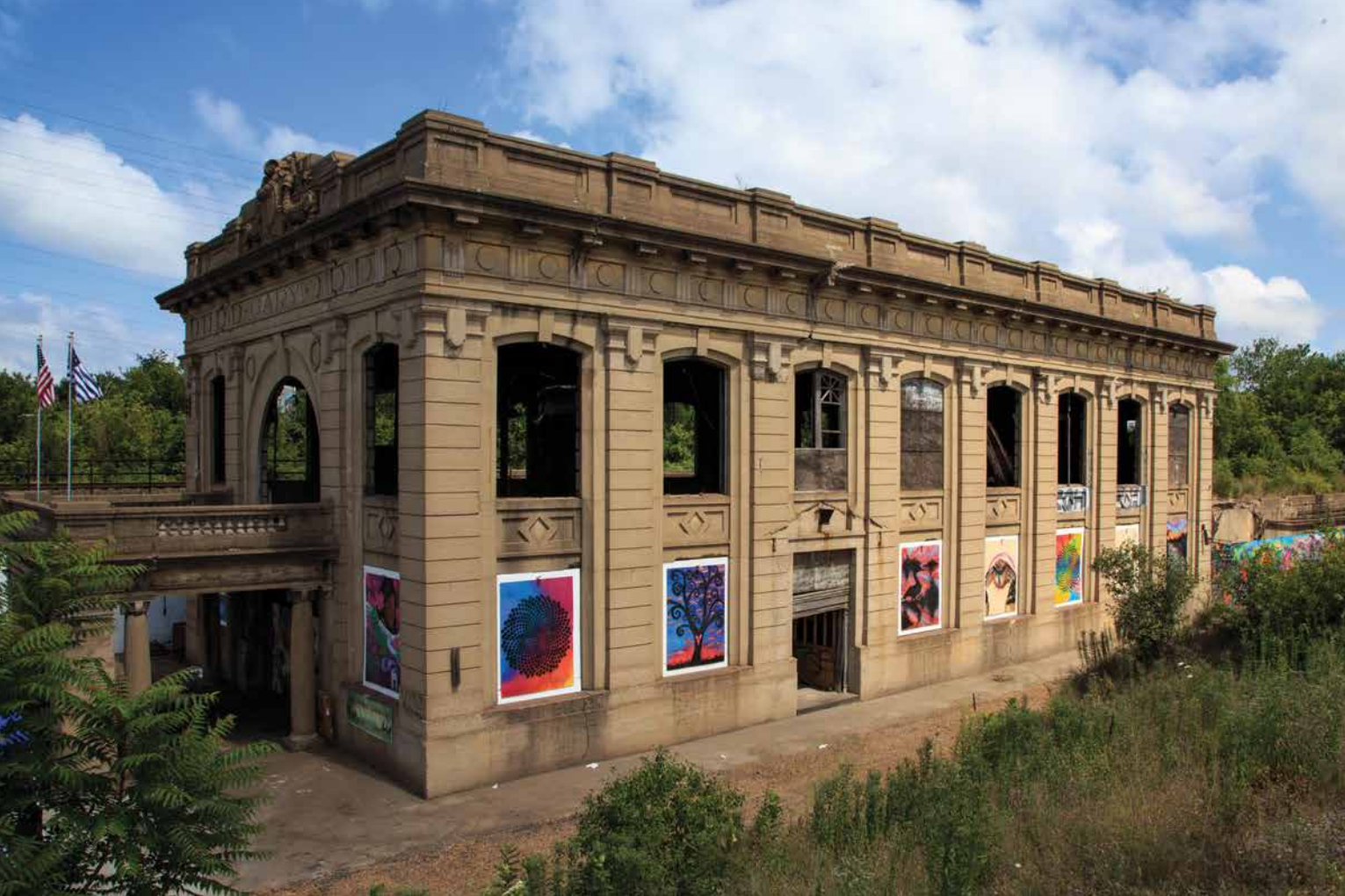
Indiana Landmarks' Efroymsen Family Endangered Places Fund makes grants to non-profits for historic building rehab and cost assessments. Last year, Gary's Decay Devils—a new affiliate—used a $3,500 grant for a structural analysis of the 1910 Union Station.
