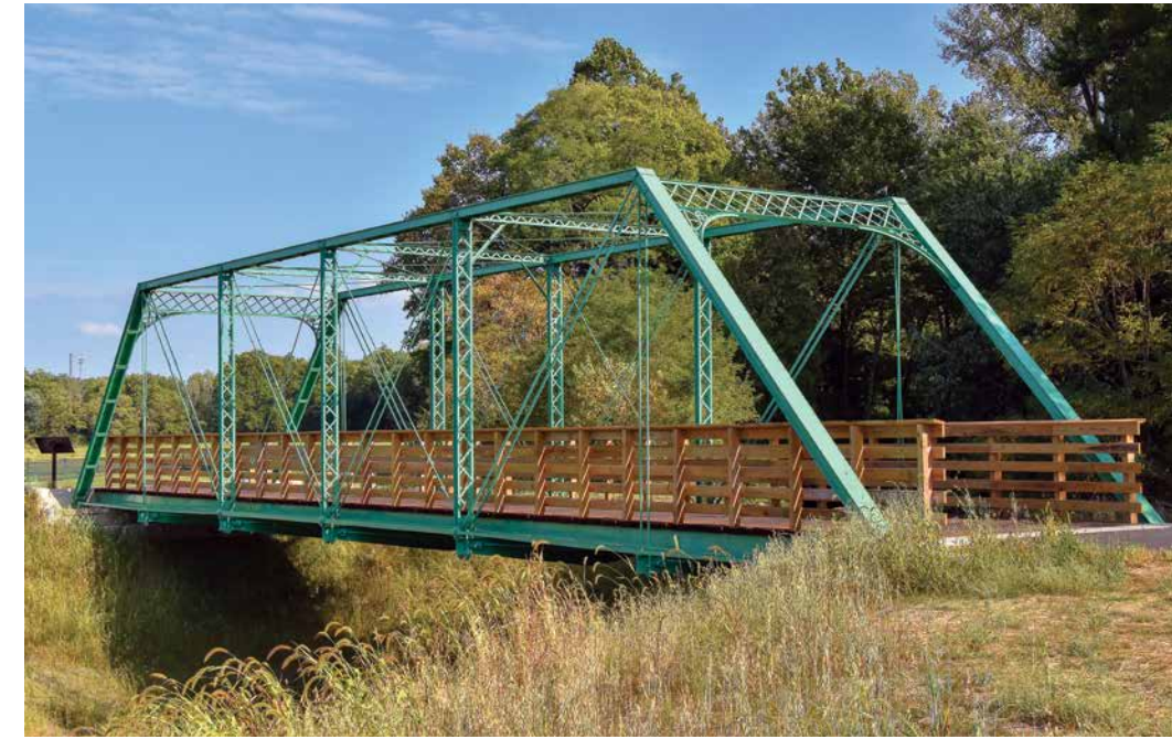
For over a decade, Indiana Landmarks encouraged rehabilitation of Shelby County Bridge #13, closed to traffic since 2011. Working with county commissioners and the state department of transportation, we helped find a solution to save the span, relocated and restored as part of a trail in Shelbyville's Blue River Memorial Park.
